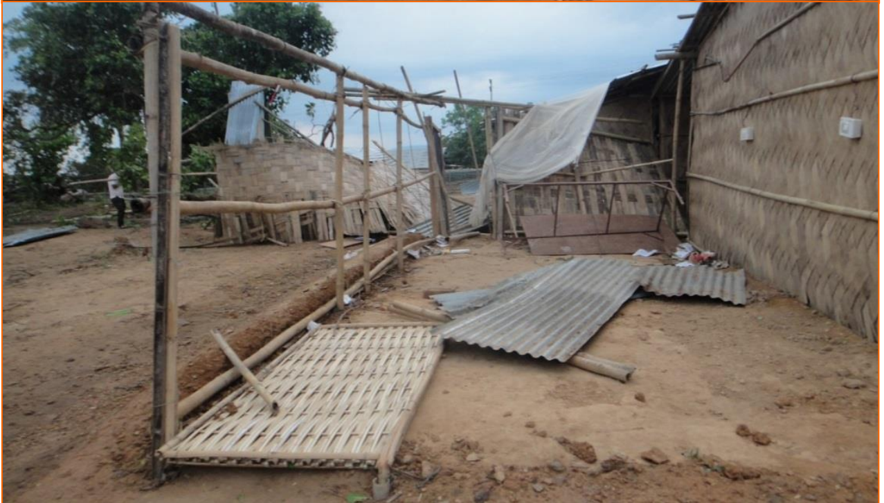
The destroyed school building
